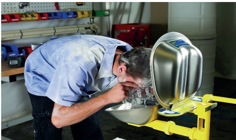
Plumbed emergency eyewash
